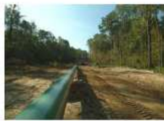
Pipeline (Source: Denbury Resources).
